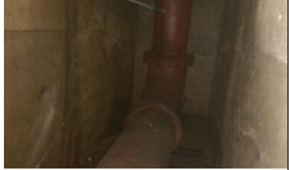
Fill line in lower pump house
