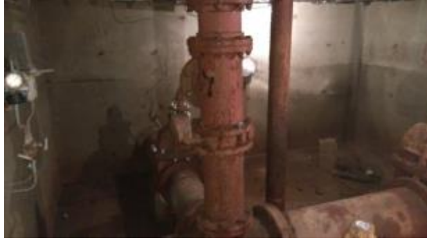
Piping in lower level of pump house
