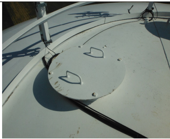
Secondary roof hatch cover
