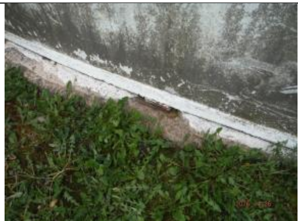
Spalling of foundation
