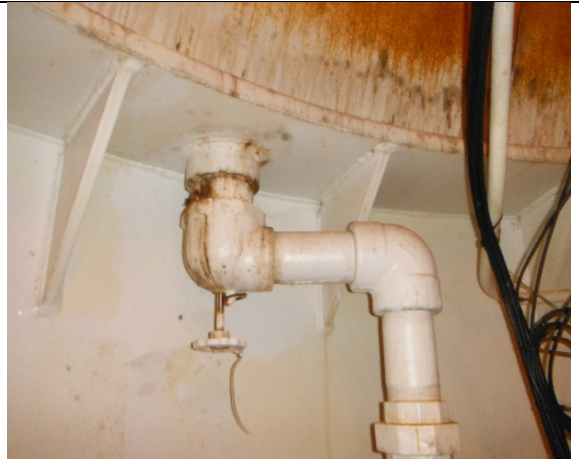
Mud valve under the inverted cone
