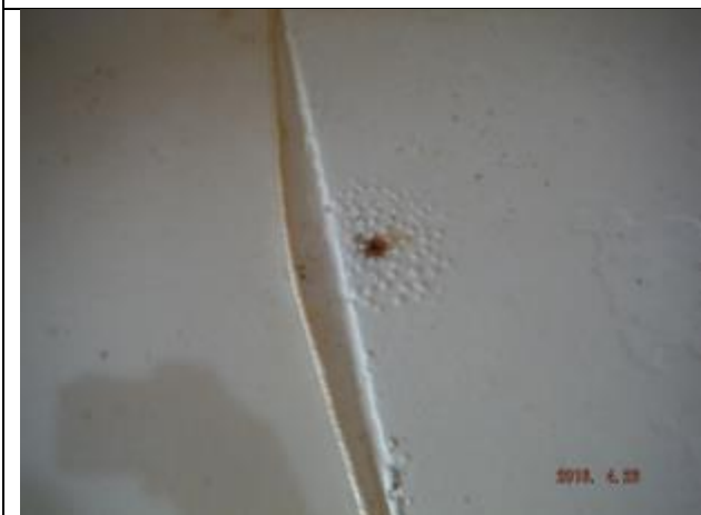
Blistering and holiday from popped blister on floor
