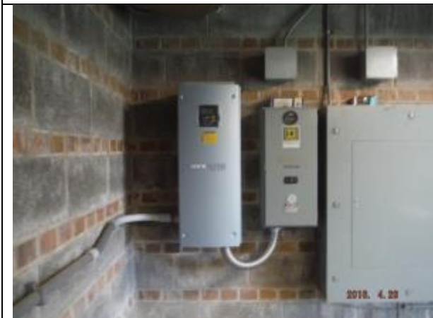
Controls in pump house
