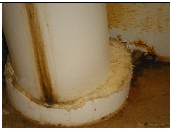
Overflow pipe in condensate platform
