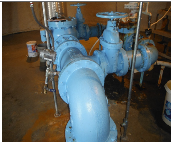
Pipes in basebell
