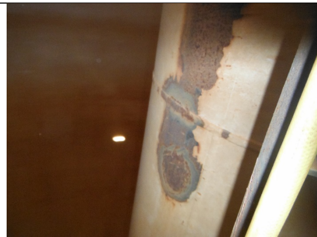
Wet interior access tube
