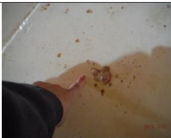
Blistering of coating on floor
