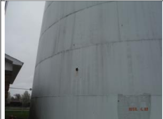
Coating break along lower exterior sidewall
