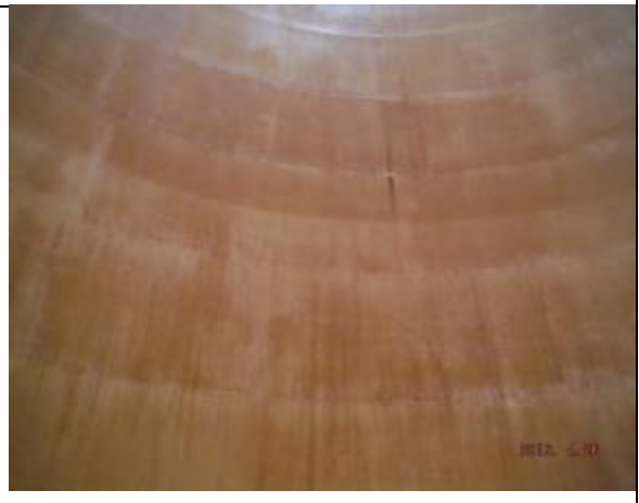
Interior sidewall. Repair of above photo can be seen near center of photo
