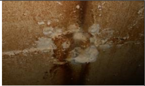
Apparent pit repair on interior sidewall seam
