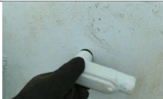
Obsolete conduit entering tank roof is loose
