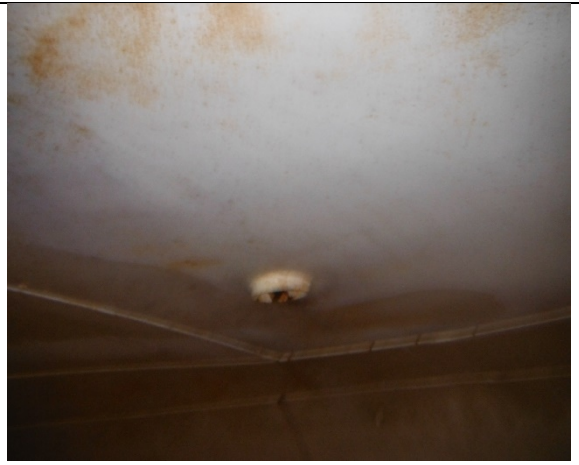
Wet interior roof
