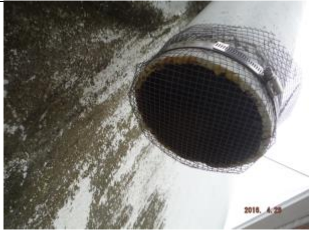
Overflow pipe screen
