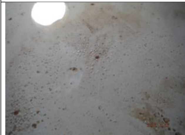
More blistering of coating on floor
