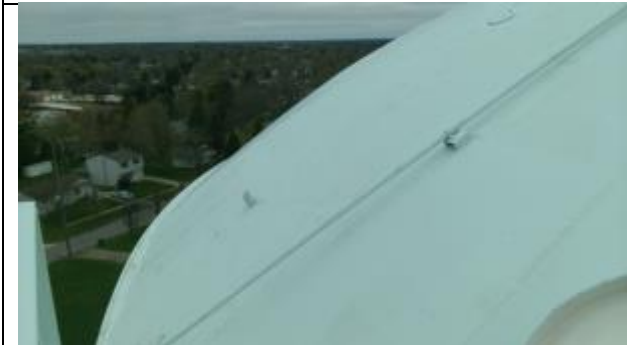
Exterior roof and obsolete conduit
