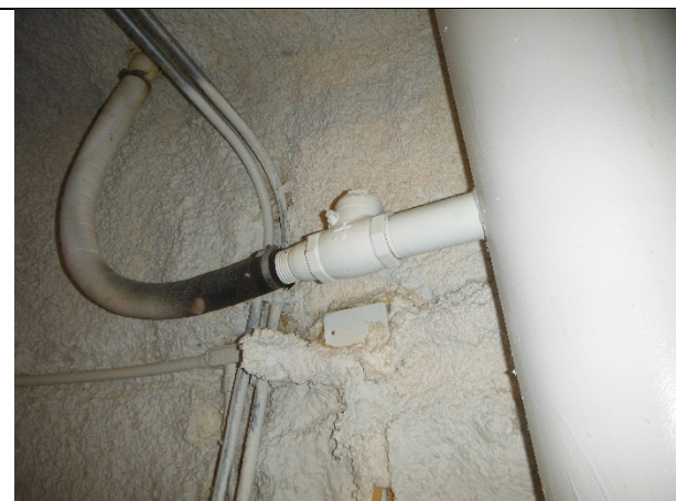
Condensate into the overflow
