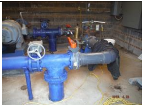
Piping on main floor of pump house
